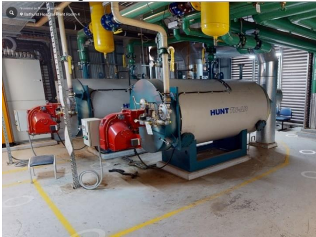
Figure 3 Heating Hot Water Generators (PR4)
