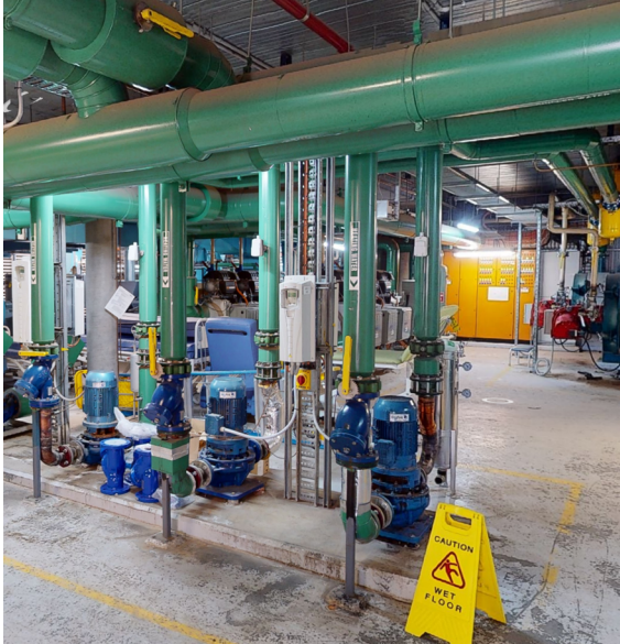
Figure 5 Heating Hot Water Pumps (PR4)
